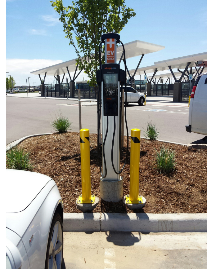
EV Charging Stations
